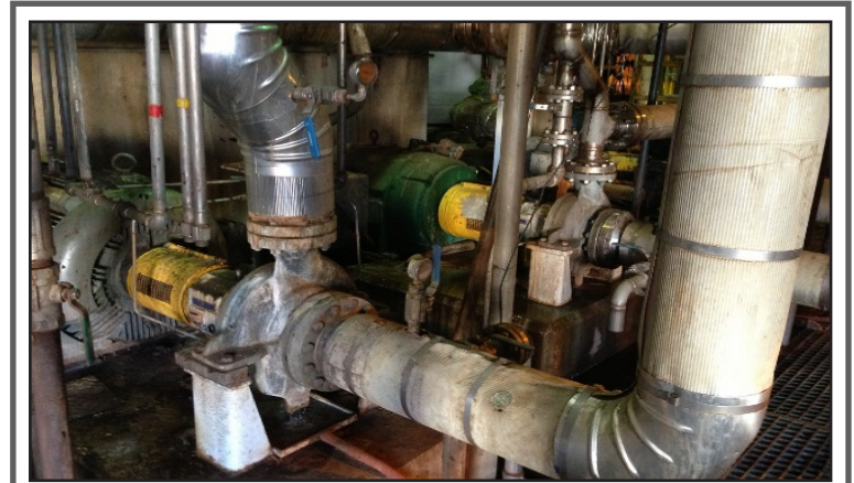
TOP: KCF sensors on digester liquor pumps;
