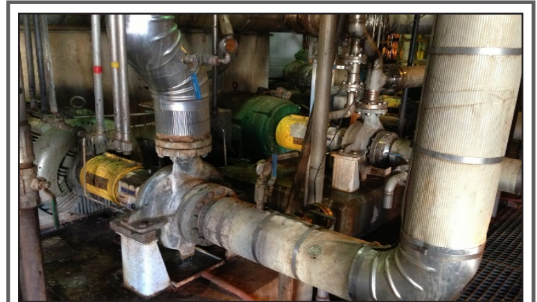
TOP: KCF sensors on digester liquor pumps;
